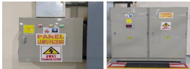
Gambar Panel Listrik
