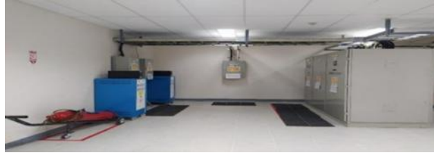
Gambar Main Distribution Panel (MDP)
